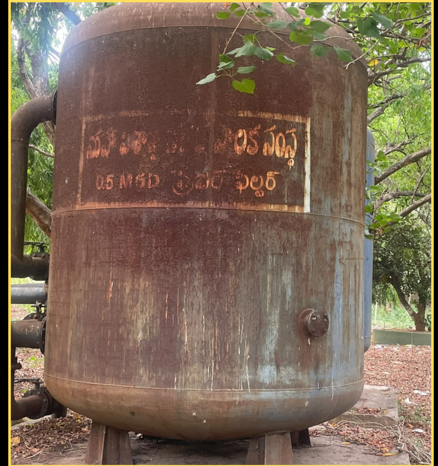
Water filter located in mudarsarlova reservoir park used for supply to Adilova and Gudisalova residents
